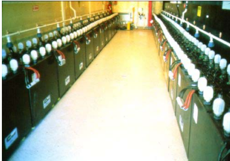
Lead acid battery bank.
