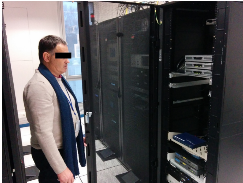
Figure 2.26: Satellite Terminals in CNES
