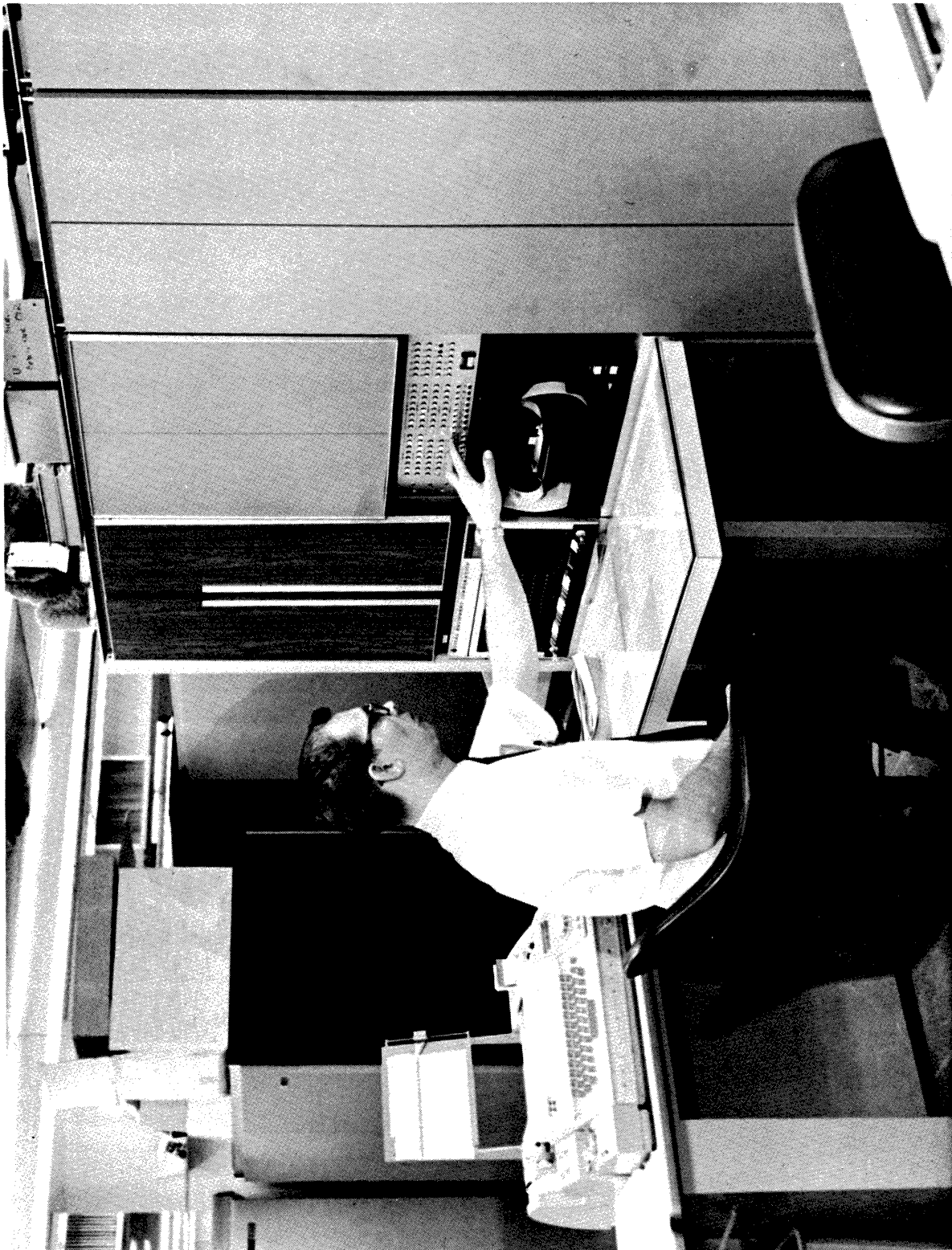
Figure i. The Data Concentrator. The Interface is in the Bay immediately above the Test Panel.
